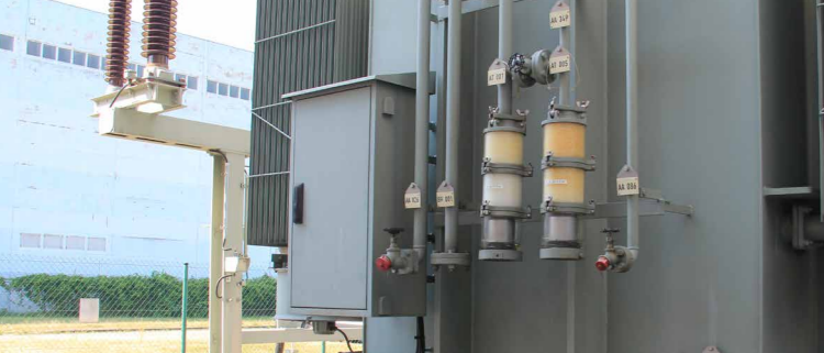
Figure 1. Typical connection and sampling field of a 40 MVA, 110 kV/15 kV transformer
