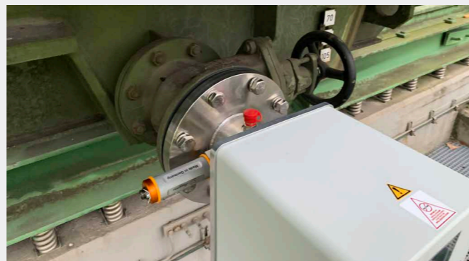
Figure 3. Direct installation on the transformer oil connections – with DGA, moisture and break-down-voltage sensors
