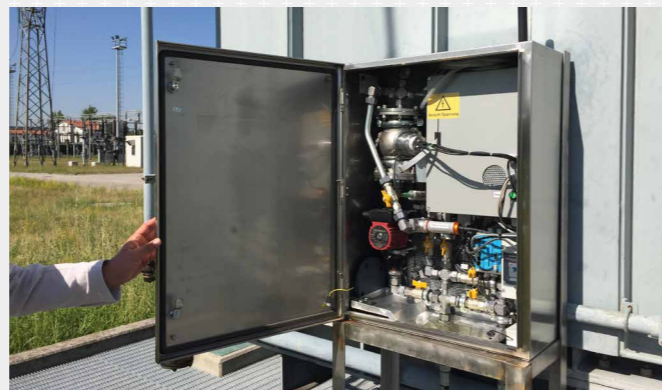
Figure 2. A bypass cabinet with oil pump and sensors
